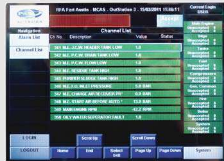
The outstation HMI has most of the features of a Workstation and can be used as a stand-alone alarm panel for smaller systems.
