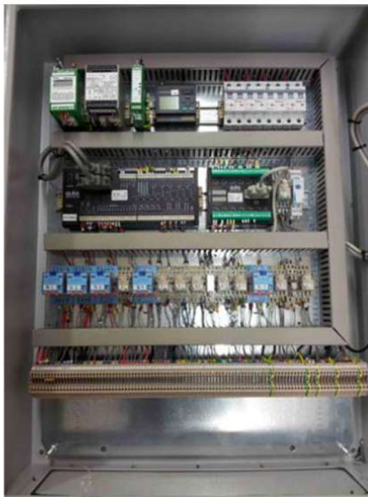
Generator Control Panel
