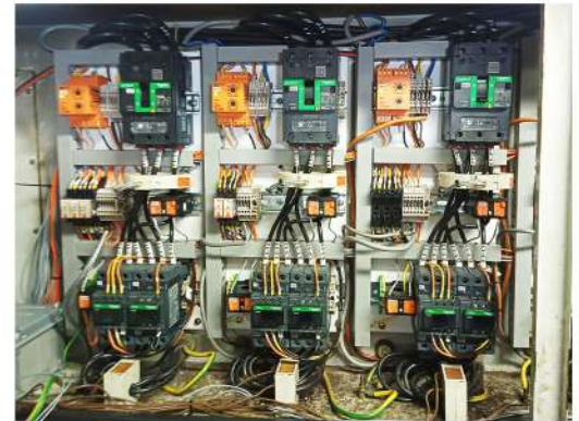
View of Starter Panel
