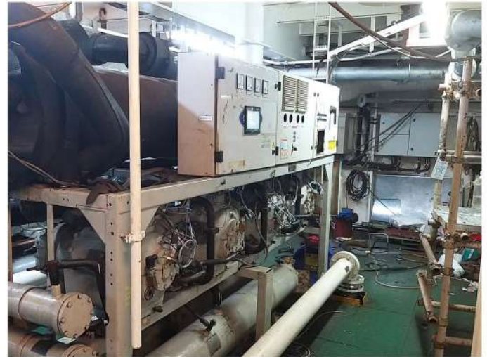
View of Carrier AC Skid
