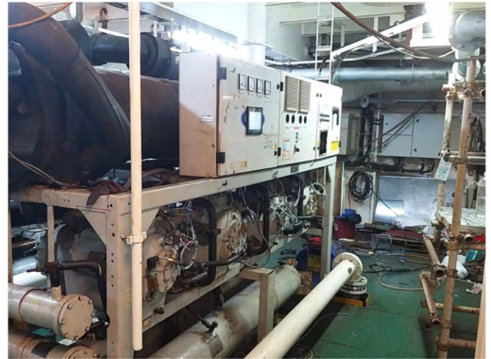
View of Carrier AC Skid
